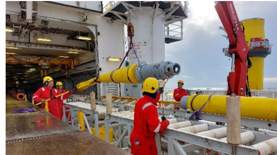
Cable Protection System (CPS) Connecting wind farm power cables
